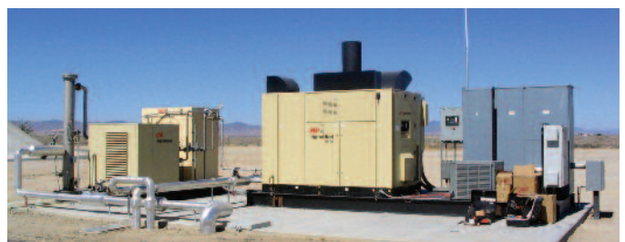
Outdoor installation of Ingersoll-Rand microturbine. Photo courtesy of Ingersoll-Rand Energy Systems
