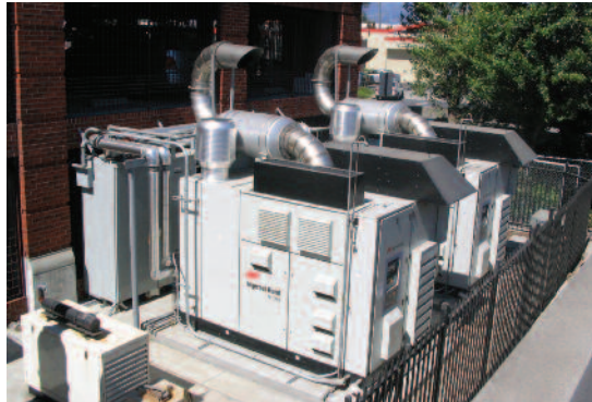
Multiple outdoor installation of Ingersoll-Rand microturbines. Photo courtesy of Ingersoll-Rand Energy Systems
