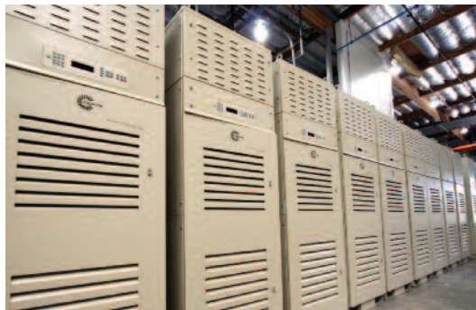
Multiple indoor installation of Capstone microturbines. Photo courtesy of Capstone Turbine Corp.
