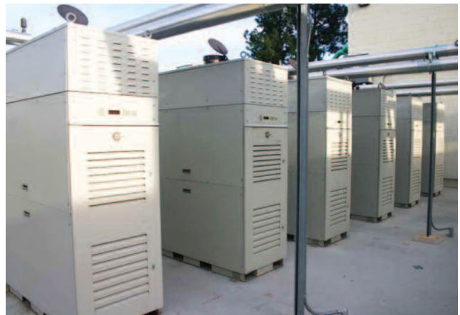
Outdoor installation of 6 Capstone microturbines. Photo courtesy of Capstone Turbine Corp.
